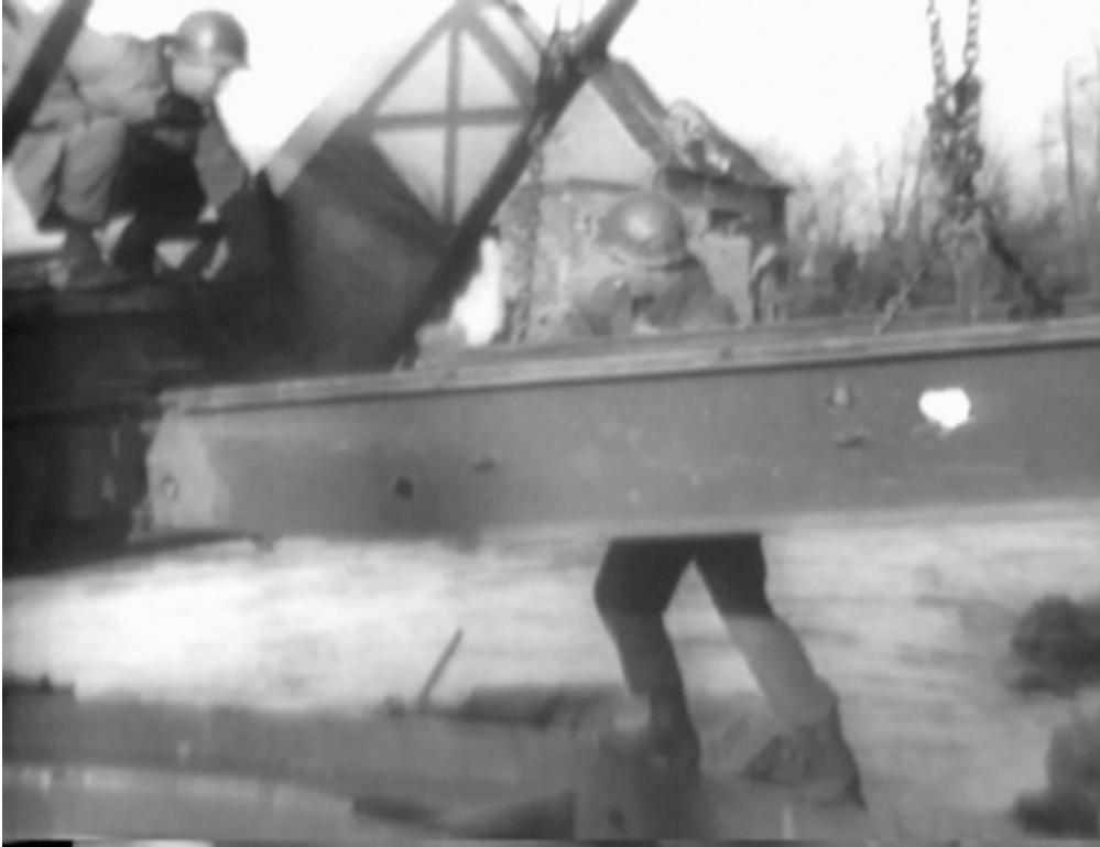
111-HRB-30_14: Combat engineers bridge the Inde River near Frenz on or about 25 November. (National Archives, Signal Corps film)
