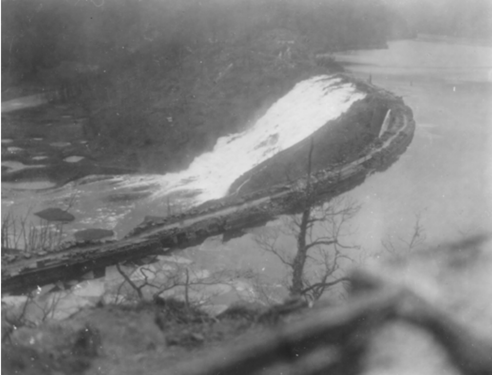
111-SC-199745: View of Urfttalsperre dam from a 9th Infantry Division OP, 5 February 1945. Craters from aerial bombing are visible below the dam, and water spills over a portion of the top damaged in an air raid. (National Archives, Signal Corps photo)
